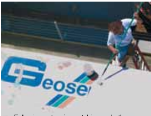
Following extensive patching and other repairs, Dora Gonzalez paints our exhibit at the Offshore Energy Center.
